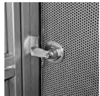
panel firmly bolted together
